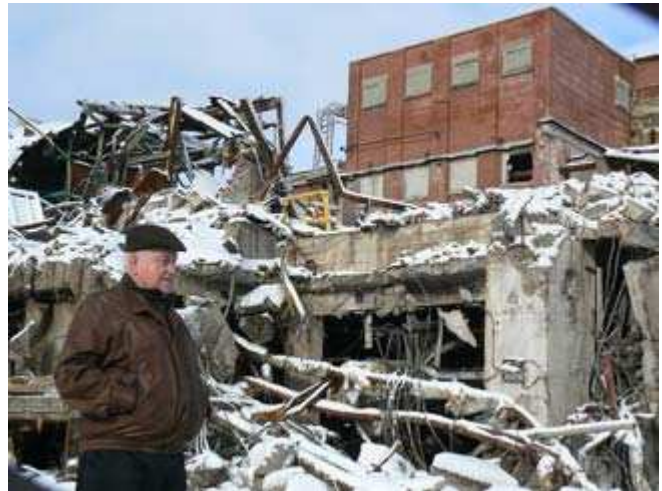
Ray Lalonde oversees demolition and decommissioning of the former Domtar site. Photo by Gary May
